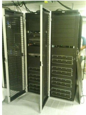
Figure 1 - Part of HPC Cluster installed at EMD
