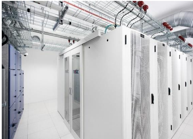
Figure 1 - Part of HPC Cluster installed at EMD
