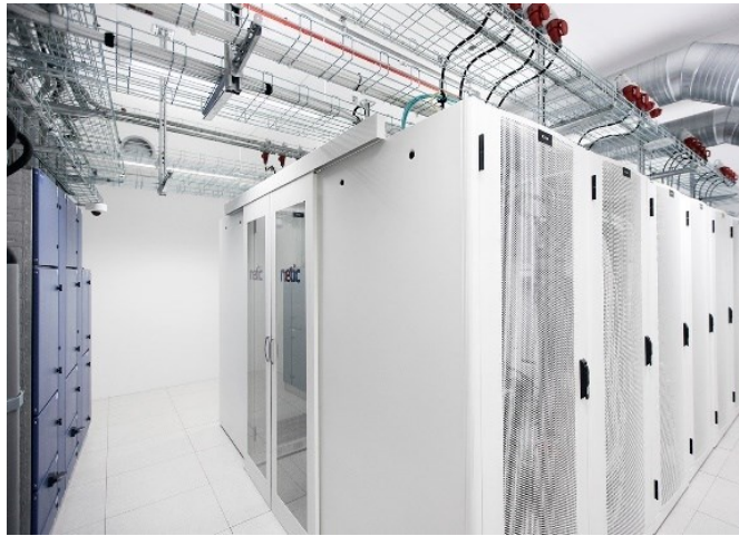
Figure 1 - Part of HPC Cluster installed at EMD
